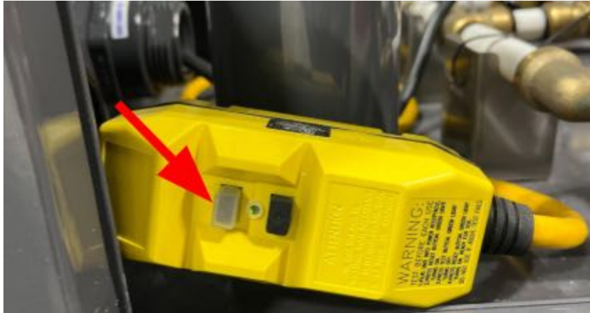
Figure 8) Turning on the GFCI Breaker
