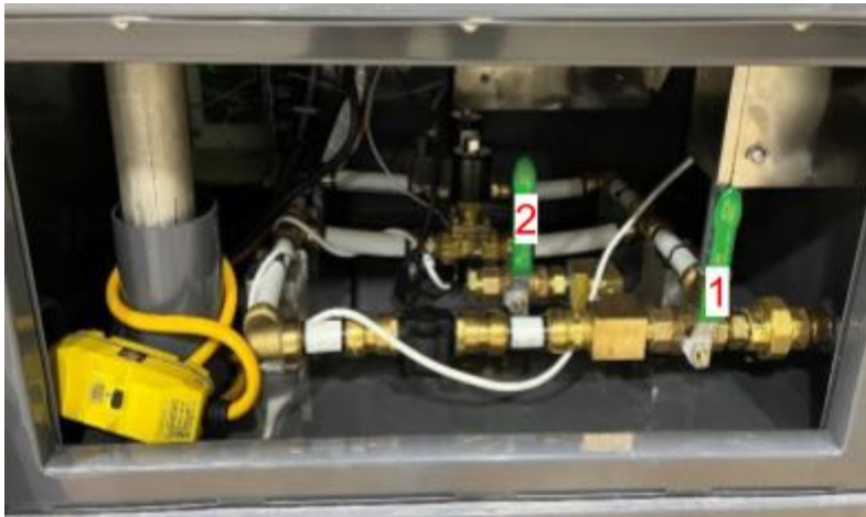
Figure 12) Open the Inlet Water Valve
